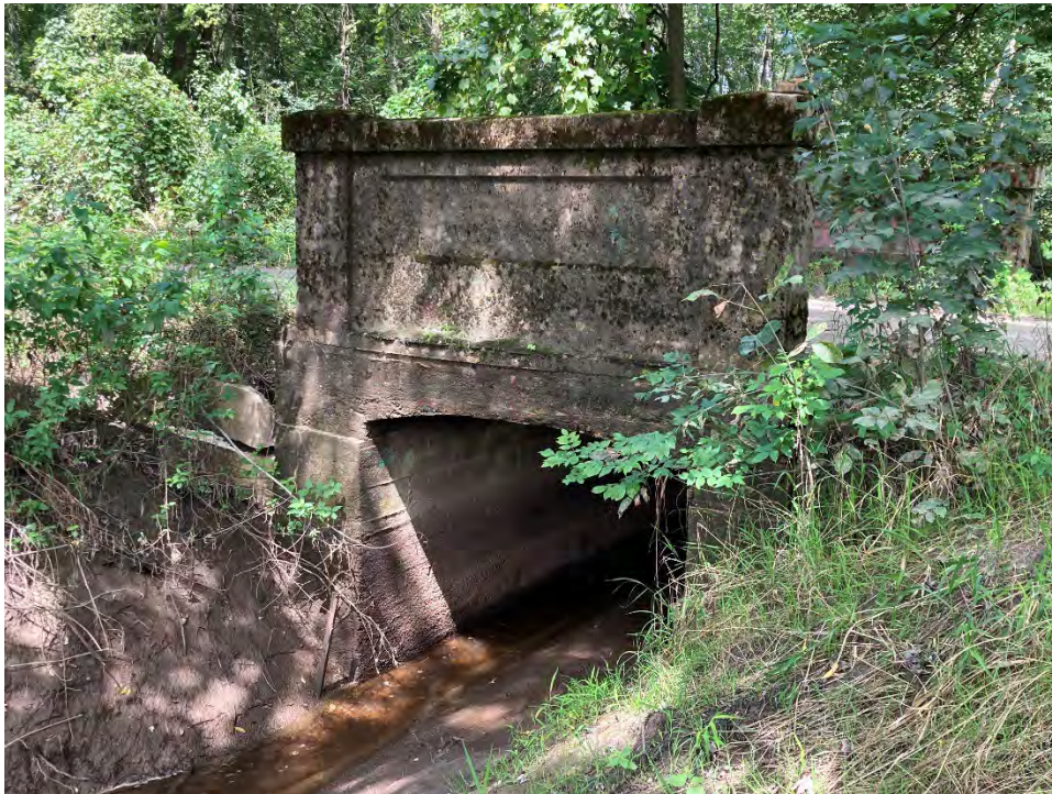
Photograph 44: Reinforced concrete culvert on Carver Street near the border of Brandon and Pittsford. Camera facing southwest.
