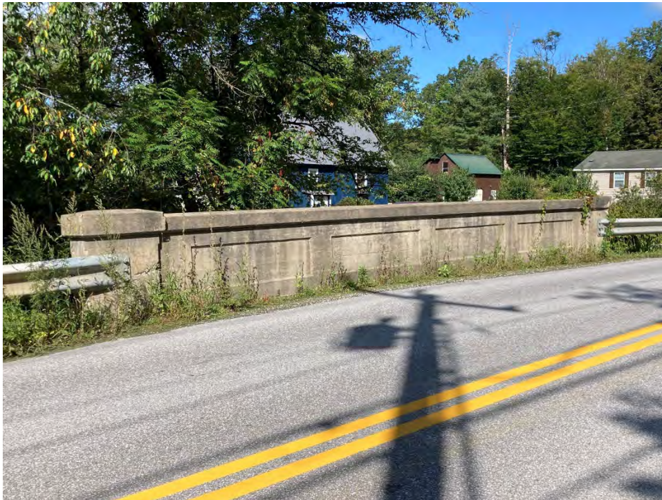
Photograph 12: The Village of Forest Dale, concrete bridge over the Neshobe River. Camera facing southeast.
