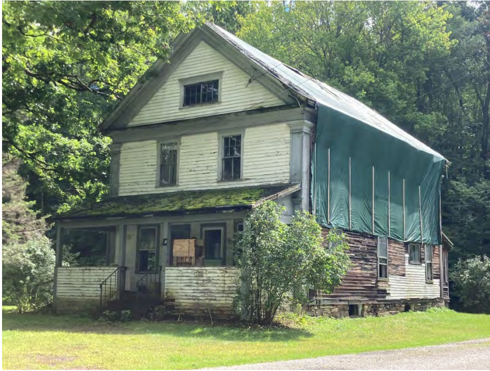
Photograph 39: The Village of Forest Dale, 45 Ray Forrest Road. SR #40. Camera facing southeast.
