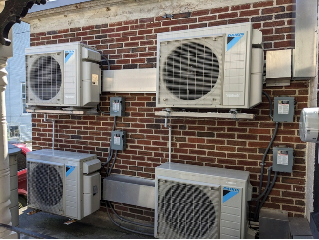
Condensers on the West Wall by the North Porch
