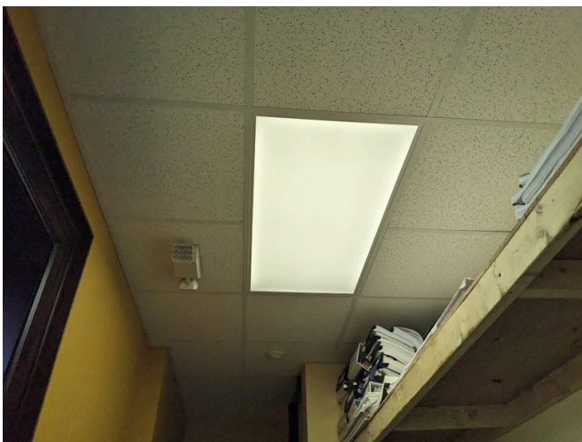
Lighting in the First Story West Hallway
