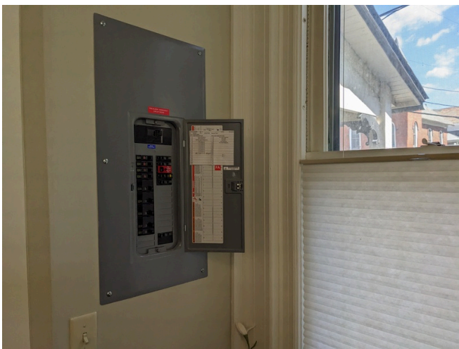
Electrical Service Panel
