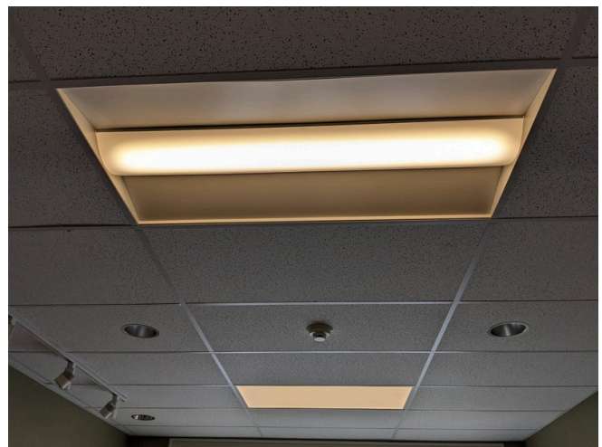
Second Story Conference Room has Three (3) Types of Lights
