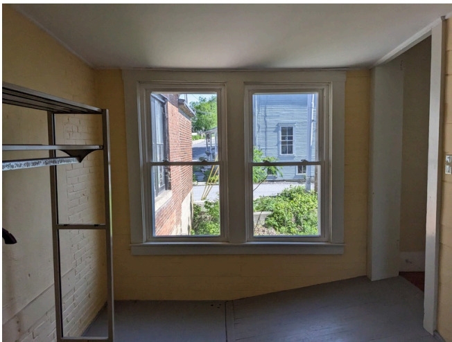
Covered Stairway Entry Shared with the Adjacent Building has a Door to the Right
