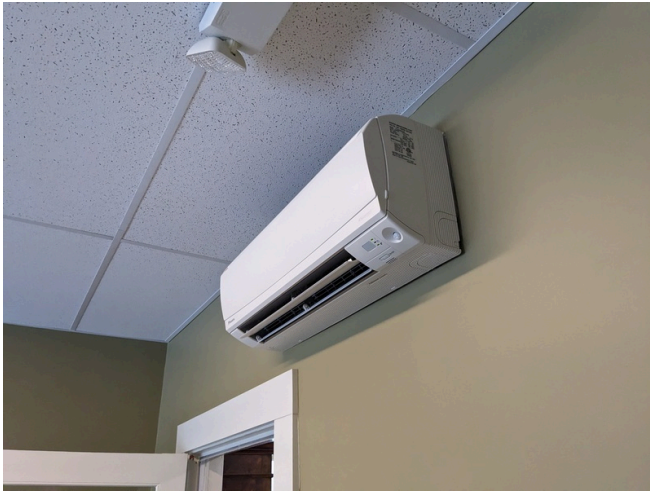
Evaporator in the Second Story South Conference Room and Office
