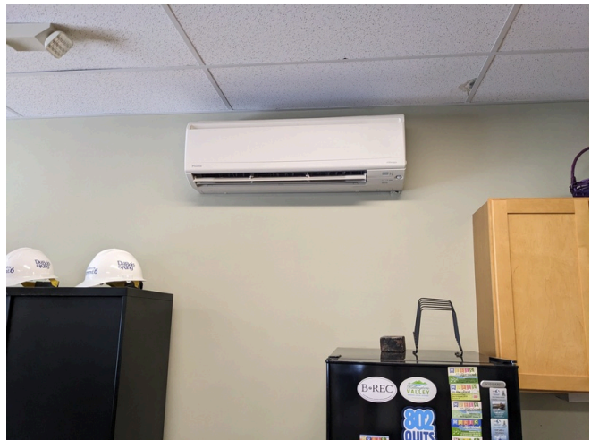
Evaporator in the Second Story Lobby
