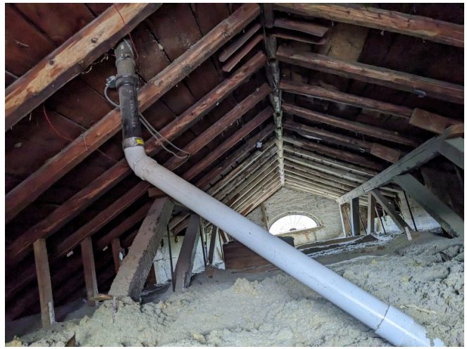
Attic Plumbing Vent
