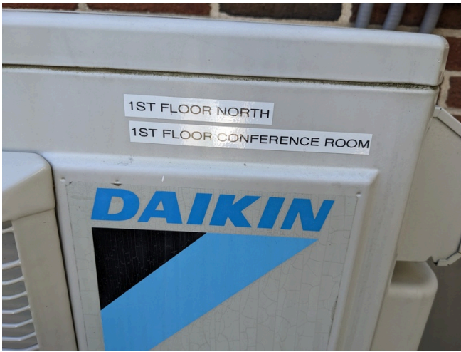
Heat Pump for the First Story North Conference Room
