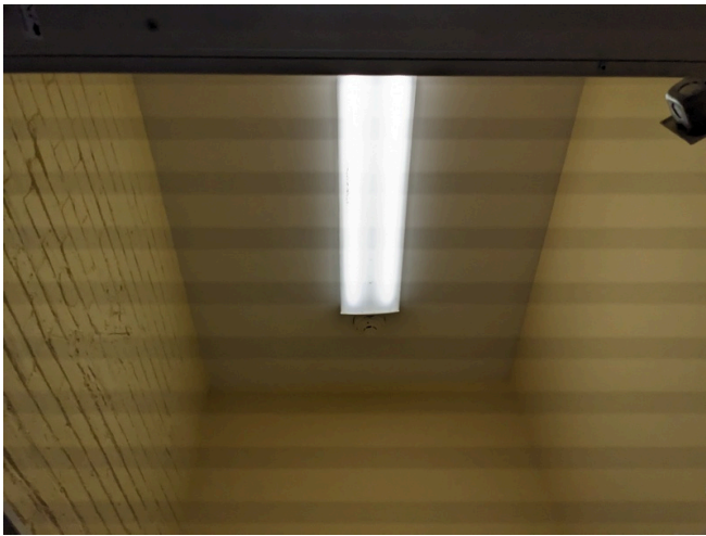
Lighting in the Shared Stairway Entry
