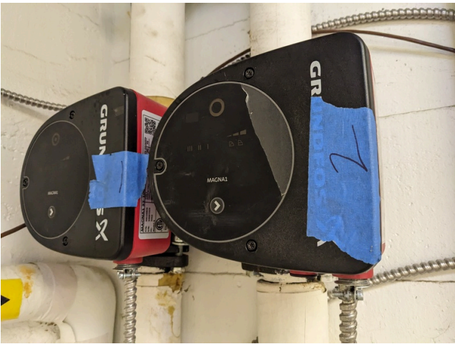
Two (2) Hydronic Pumps by Grundfos
