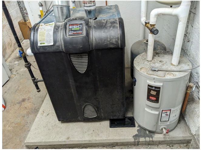
DHW and Hydronic Boiler
