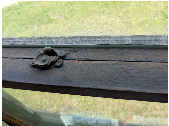
First Story West Window Lock is Broken
