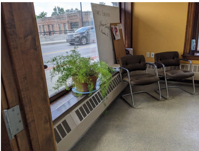
First Story Hydronic Baseboard Heaters
