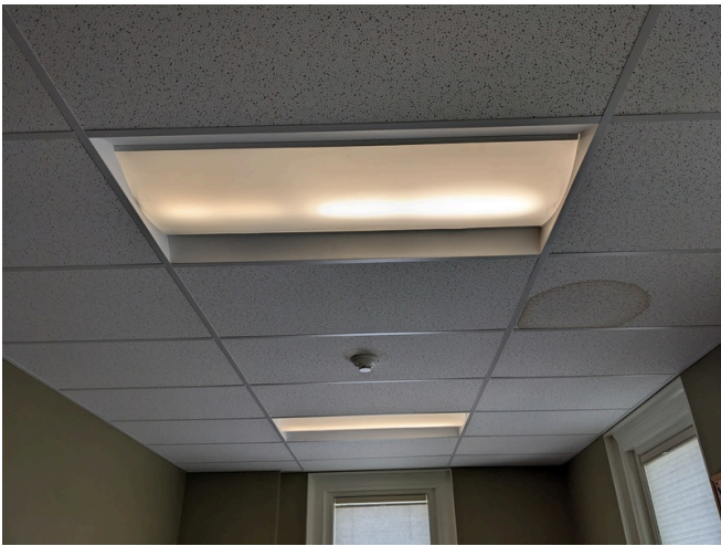
Lighting in the Second Story Office
