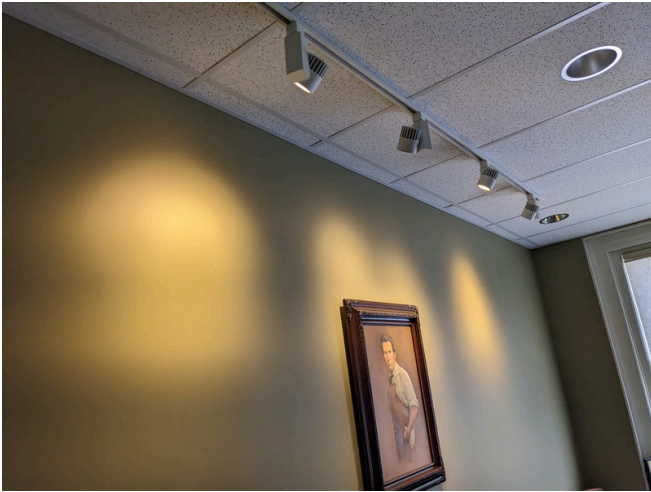
Track Lighting in the Second Story Conference Room
