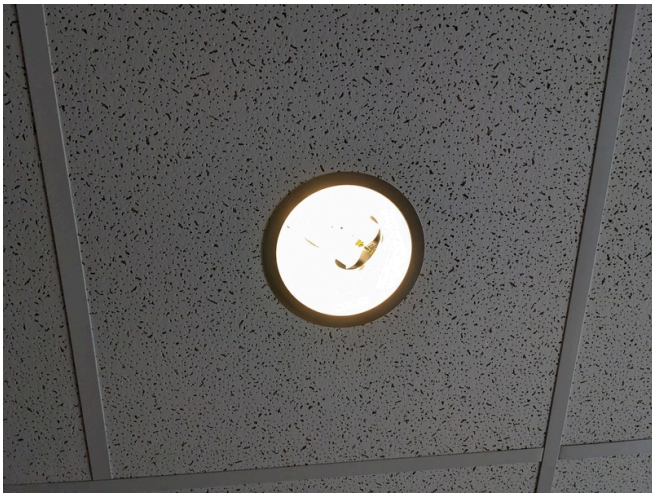
Lighting CFL in Recessed Can
