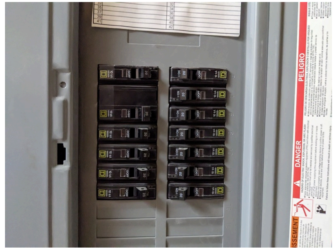
Electrical Sub Panel
