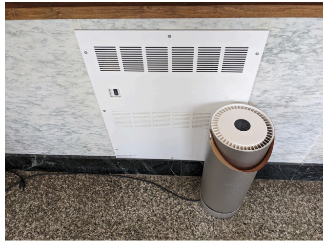
Heating Units in the First Story Service Counter
