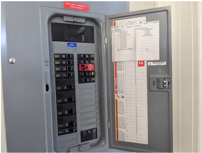
Electrical Service Panel
