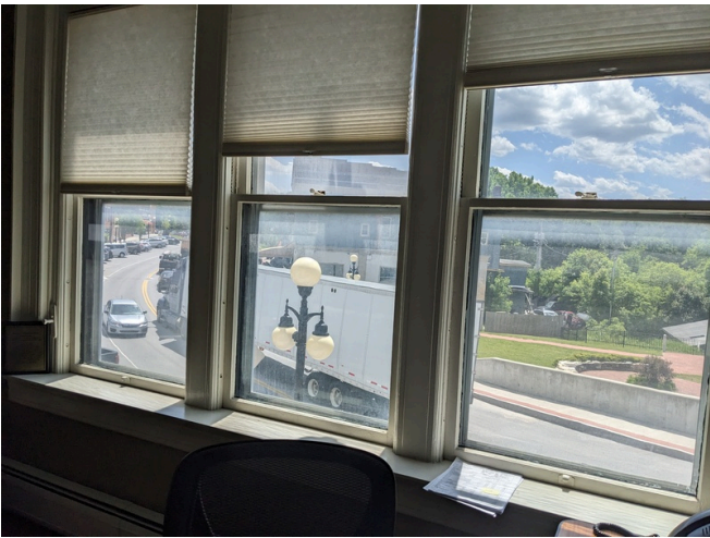
South Windows Traffic Noise and Pollution Intrusion
