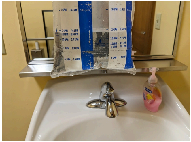
1.8 GPM Measured Flow at a Restroom Faucet
