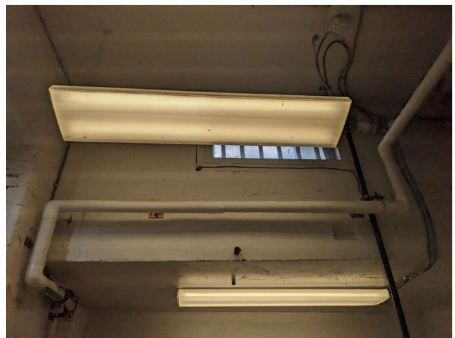
Lighting in the Mechanical Room
