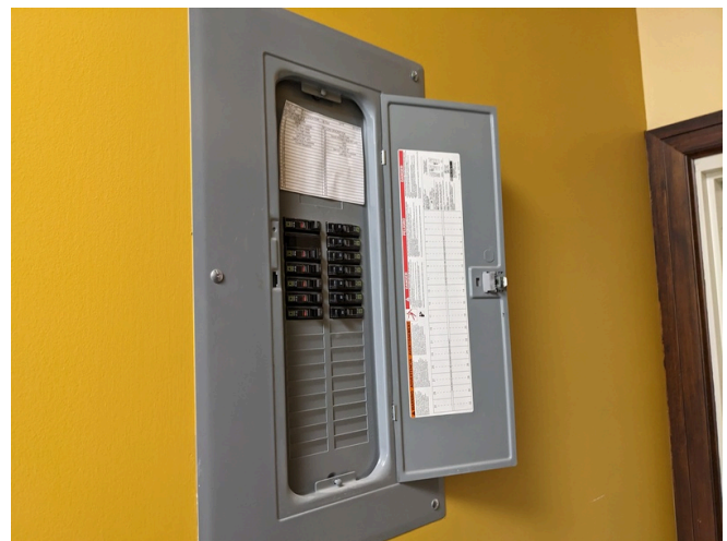
Electrical Sub Panel in the First Story West Wall
