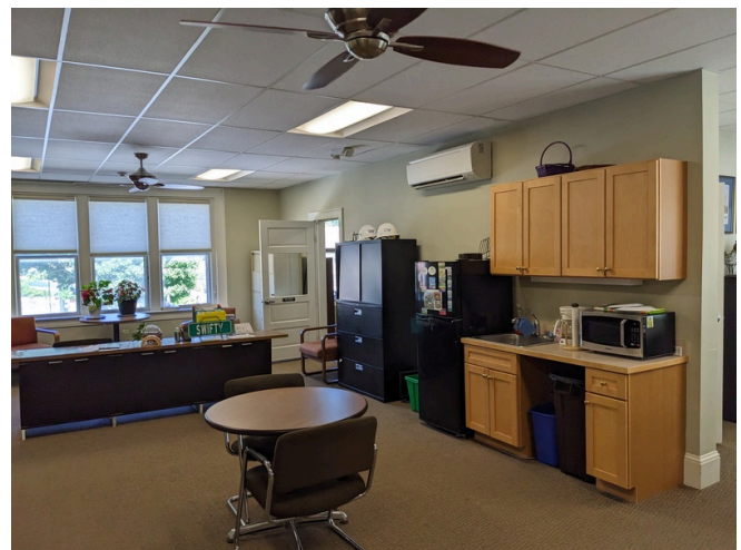
Second Story Lobby Kitchenette has an Evaporator
