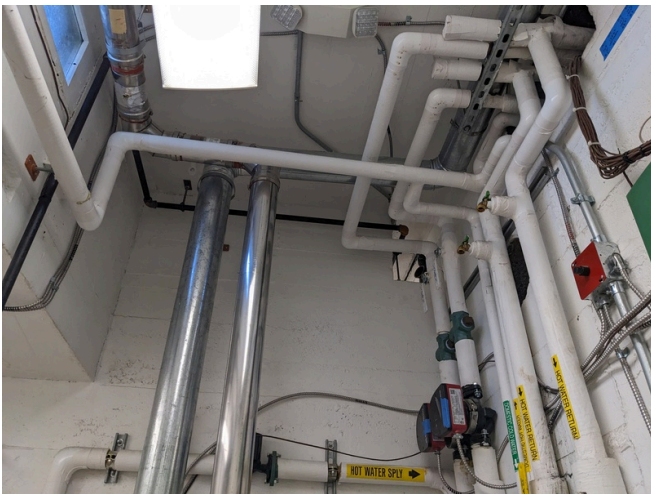
Flue and Plumbing
