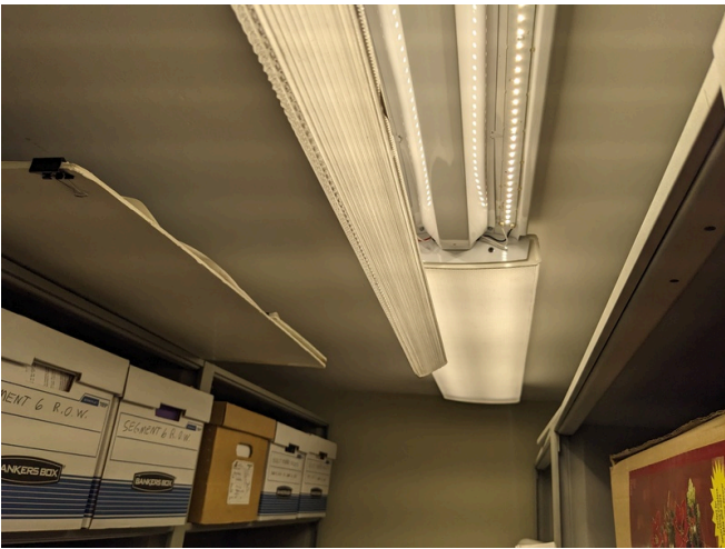
LED Lighting in the Record Vault
