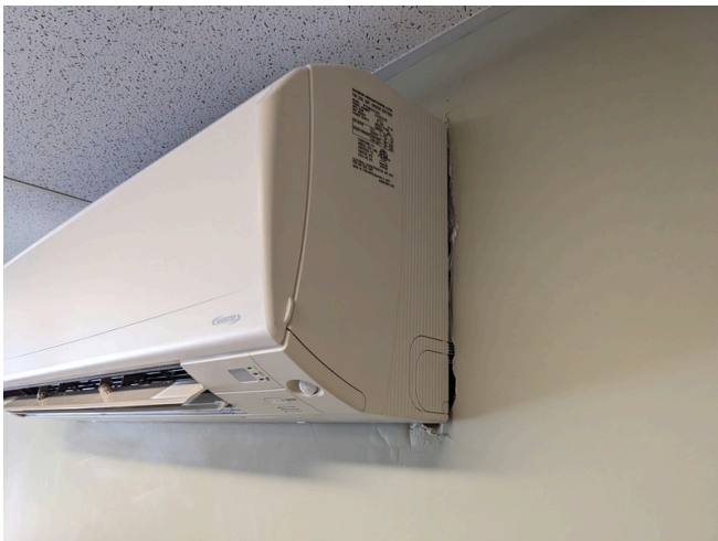
Hole in the Wall Around Evaporator Installation
