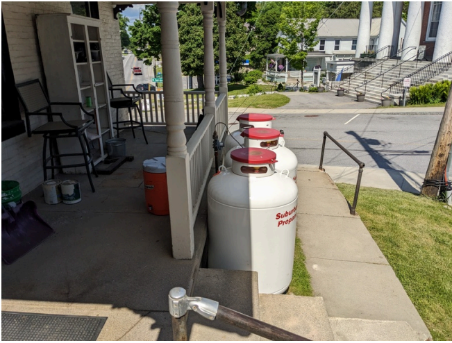
Three Propane Tanks
