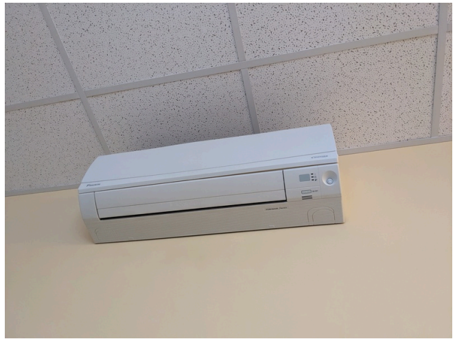
Evaporator in the First Story Northeast Corner Conference Room
