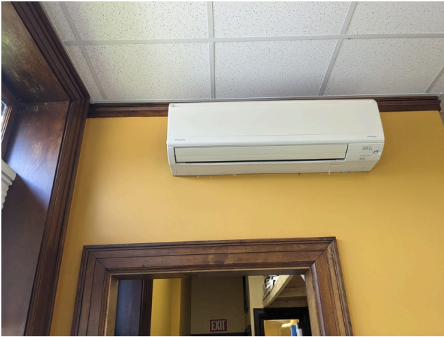
Evaporator in the First Story Southwest
