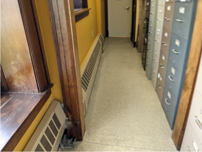
First Story West Wall Hallway Hydronic Baseboard Heater
