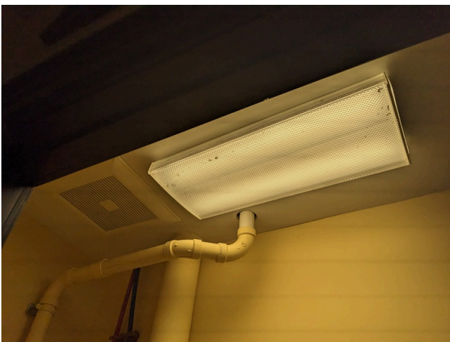
Lighting and Exhaust Fan in the Housekeeping Closet
