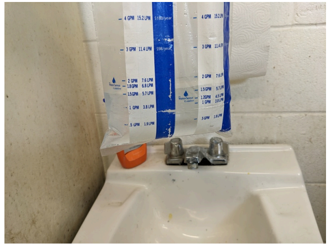
1.5 GPM Measured Flow at the Restroom Faucet in Building One (1)
