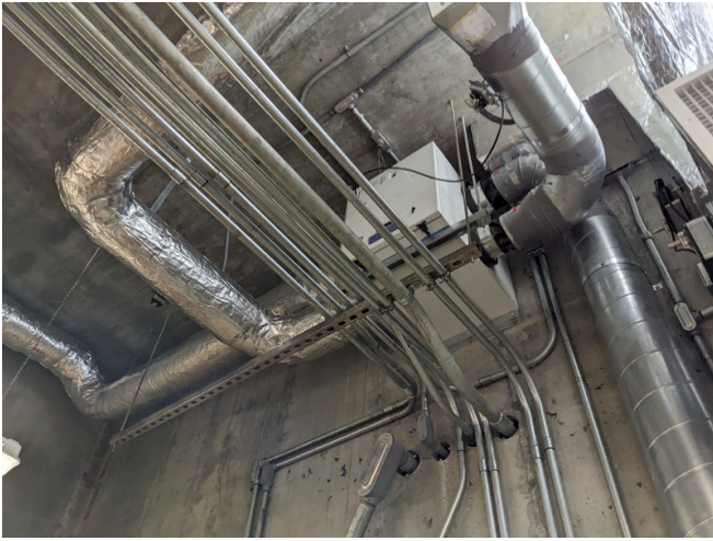
New Pond Pump Room ERV
