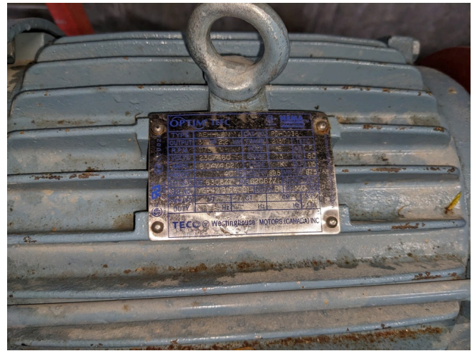
3 HP Pump for the New Pond is Insufficient So, the spare pump from the other building is being used as the primary here.
