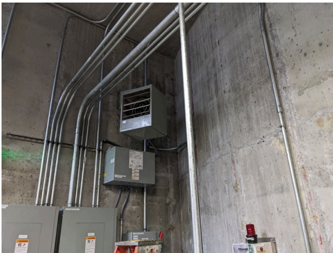
New Pond Pump Room Heater
