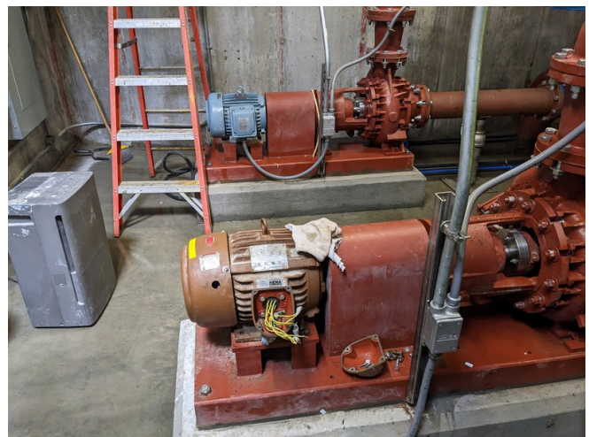
Two Pumps for the New Pond
