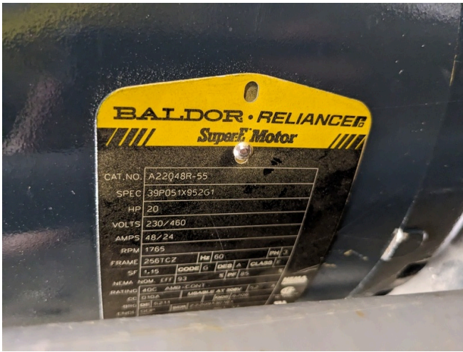
20 HP in the B1 Pump Room
