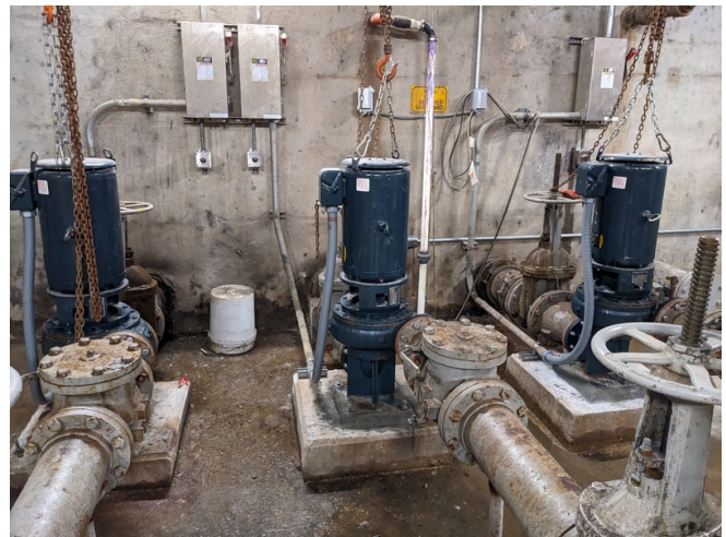
B1 Basement is the First Pump Room
