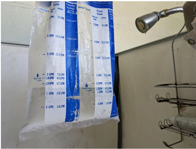
1.2 GPM Measured Showerhead in Building 1
