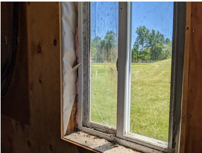
B4 South Wall Window is Broken
