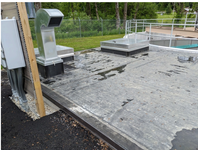
B6 is a Flat Black Rubber Roof, One Vent and Two Access Hatches
