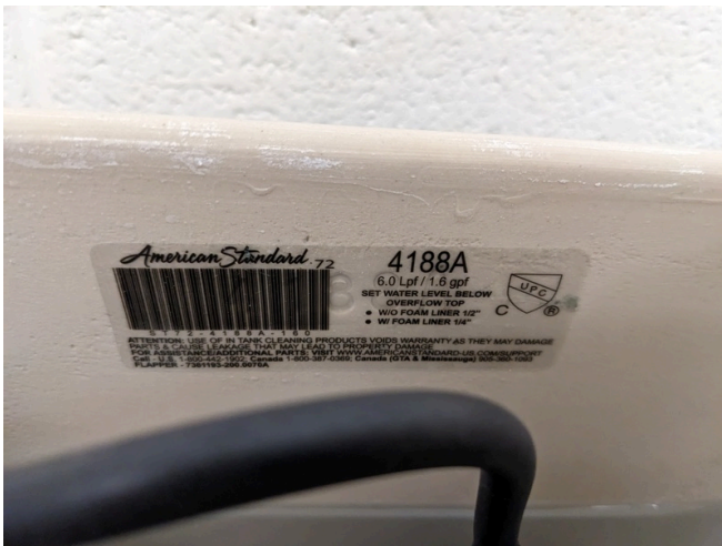
1.6 GPF Toilet in Building One (1)
