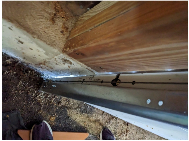
B4 Garage Overhead Doors
