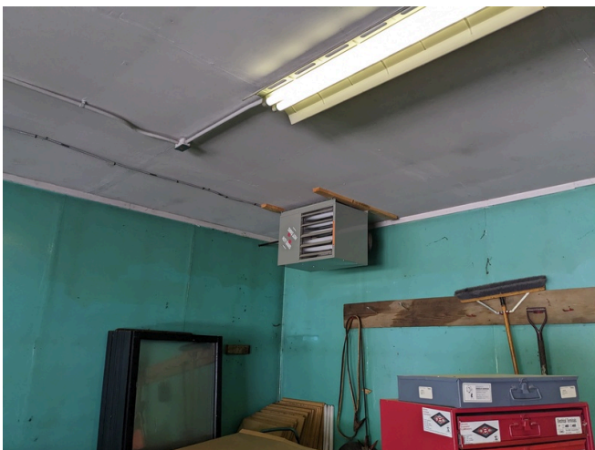
B5 Garage Heater is a Modine Hot Dawg with No Label
