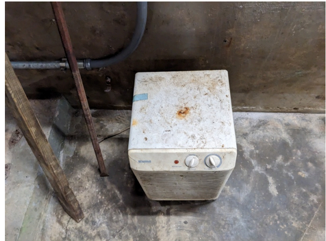
B1 Dehumidifier in the Basement
