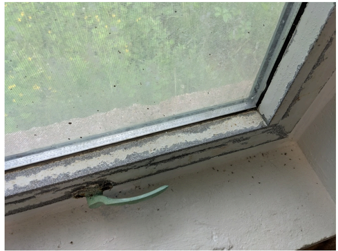
B3 Window Double Glazed Metal Frame and Handle are Oxidizing
