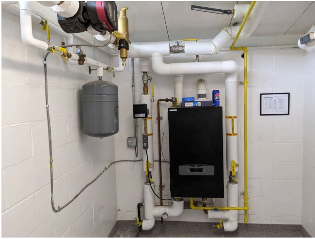
B1 Hydronic Boiler
