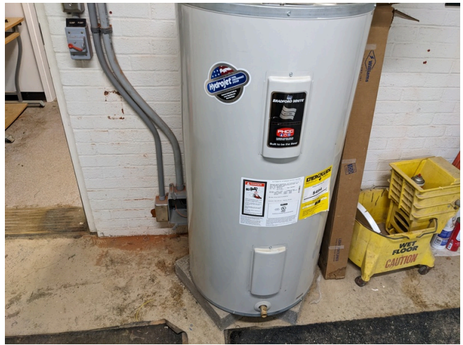
DHW in Building #2
