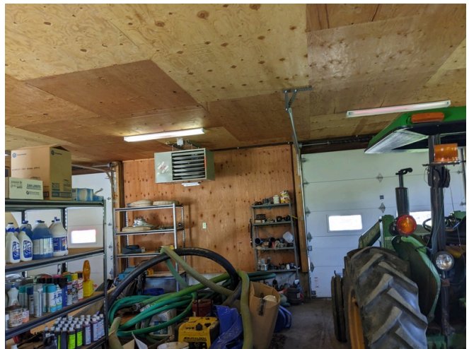
Building Four (4) Lighting
