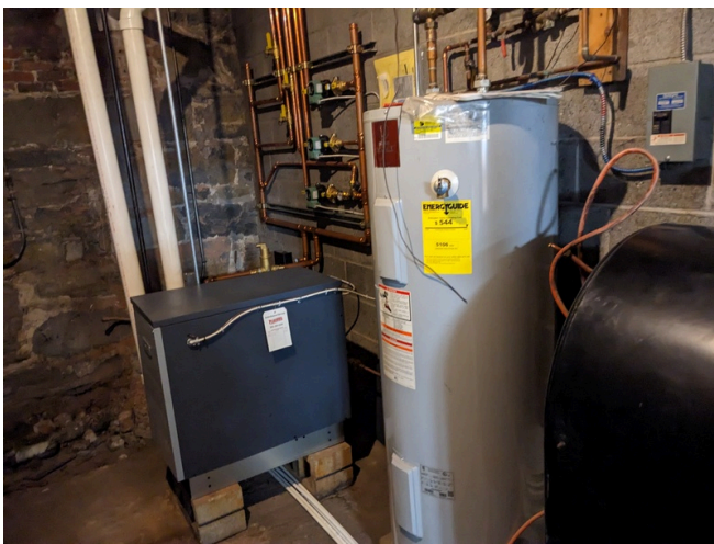
Hydronic Boiler and DHW Tank in the Mechanical Room
