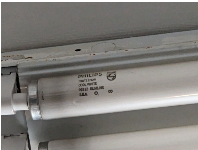
Lighting 96 W Eight Foot T12 LF
