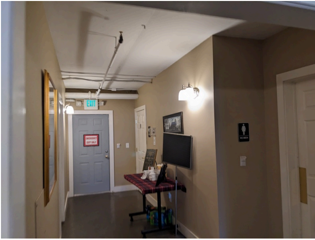
Lighting Wall Scone First Story Hallway of Restrooms; Looking East
