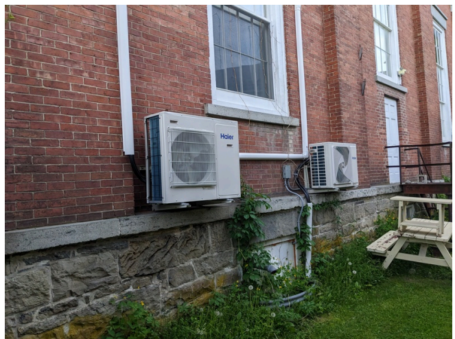
ASHP Condensers on the East Wall
