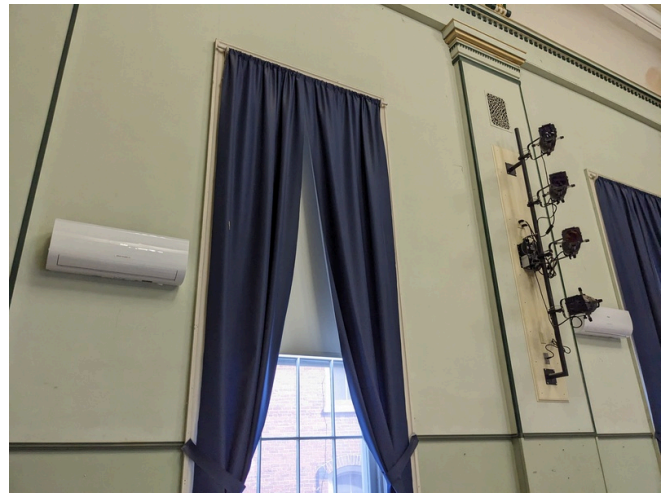
Second Story ASHP Evaporators, Window Shades and Curtain, Wall Vents and Theater Lighting
