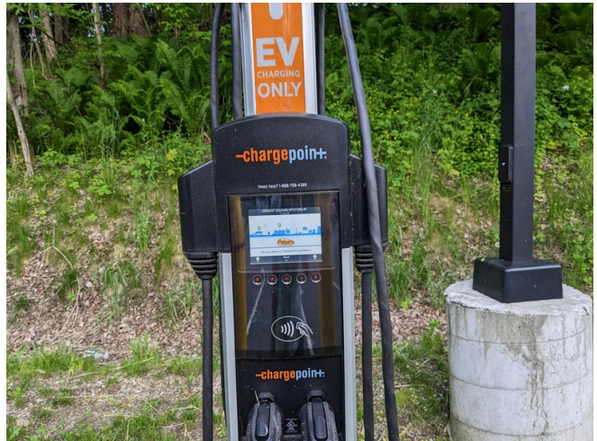
EV Charge by Chargepoint
