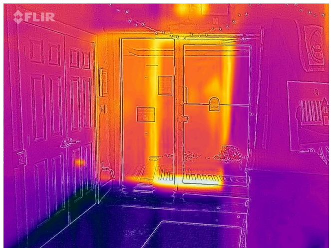
IR First Story West Wall Store Front Glass Main Entry Door and Window
