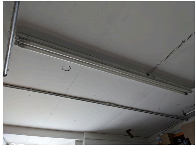
Eight Foot T8 Linear Fluorescent Lamps
