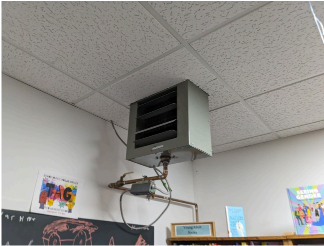
Hydronic Coil by Modine with Zero Clearance from Acoustic Drop Ceiling in the Back of the First Story Hall Temporary Library
