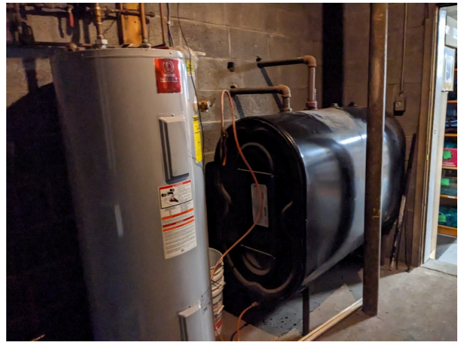
Mechanical Room DHW and Oil Tank
