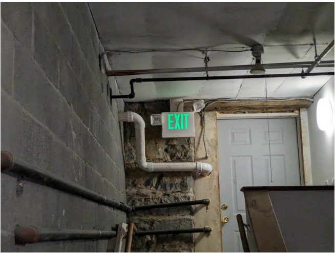
Plumbing and Vents by the First Story West Back Door
