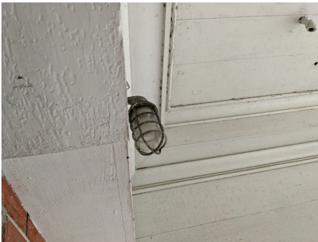
Lighting in the Front Overhang at the Third Story Exit
