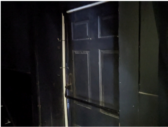
Second Story East Back Exit Door is Very Drafty
