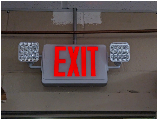
Illuminated Exit Signs with Strobe Lights
