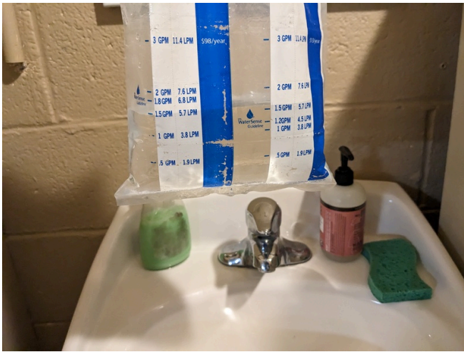
1.5 GPM Measured at the Private Restroom Faucet
