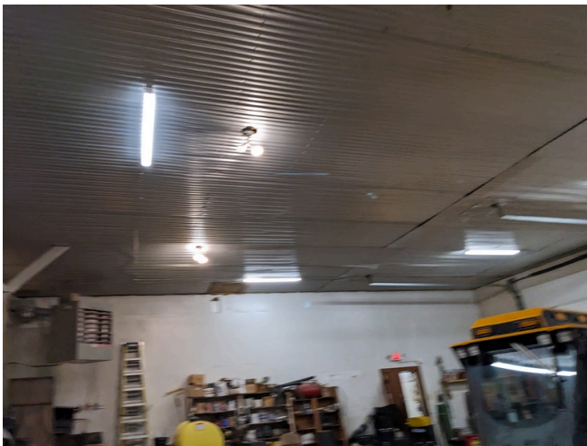
New - West Room Lighting
