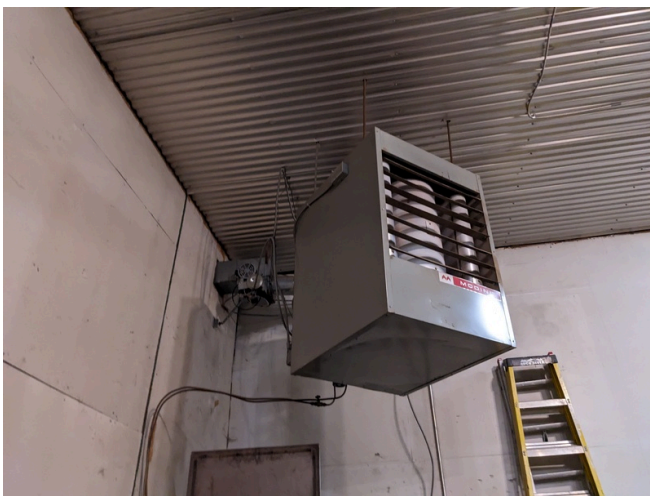
New - Ductless Furnace by Modine in the West Room of the New Building
