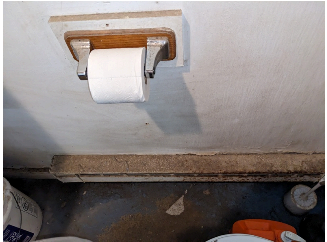
New - Restroom Baseboard Heater
