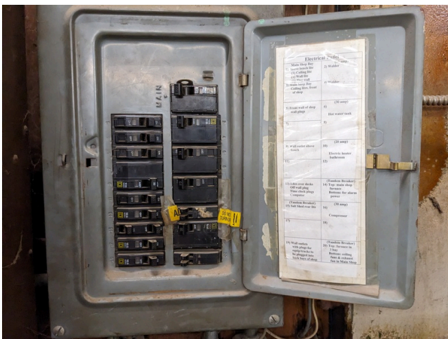
New - Electrical Service Panel
