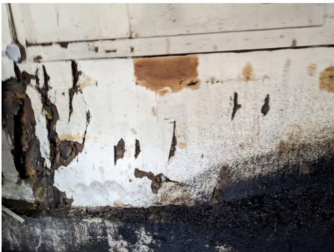
Old - East Wall has Holes
