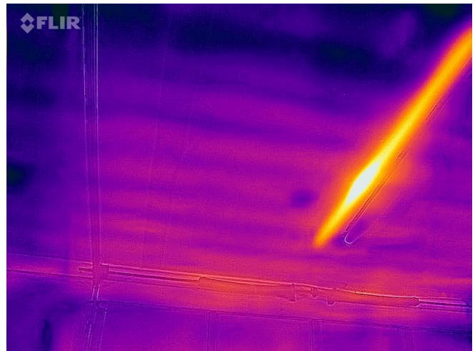
New - IR East Room Ceiling
