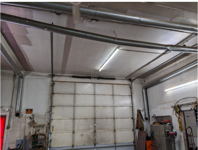
New - East Room Lighting
