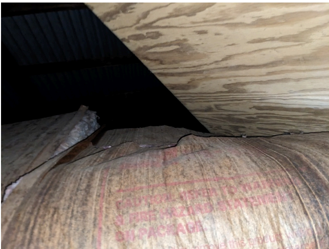
New - Attic Fiberglass Batt Insulation
