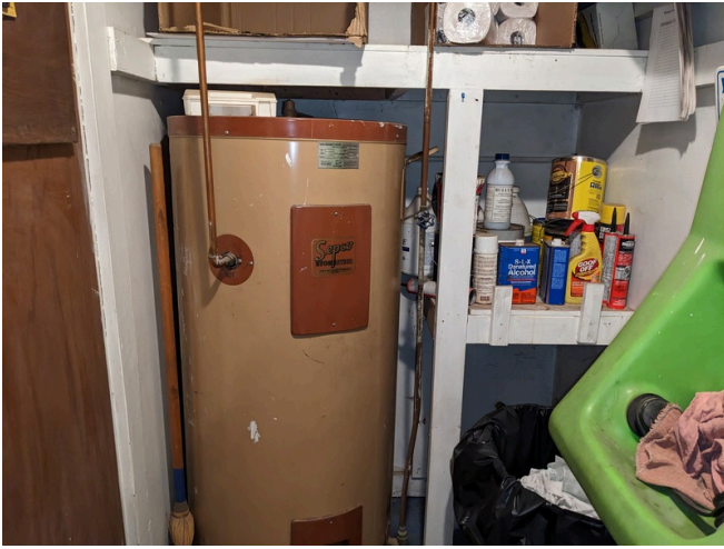
New - DHW in the Restroom
