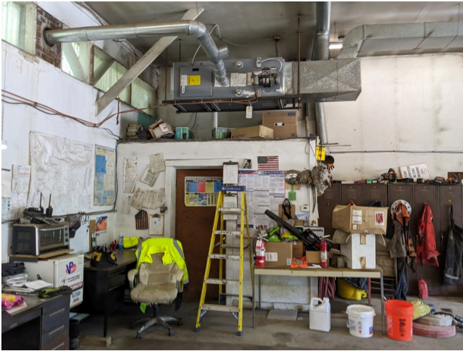
New - East Wall; Furnace Above the Restroom
