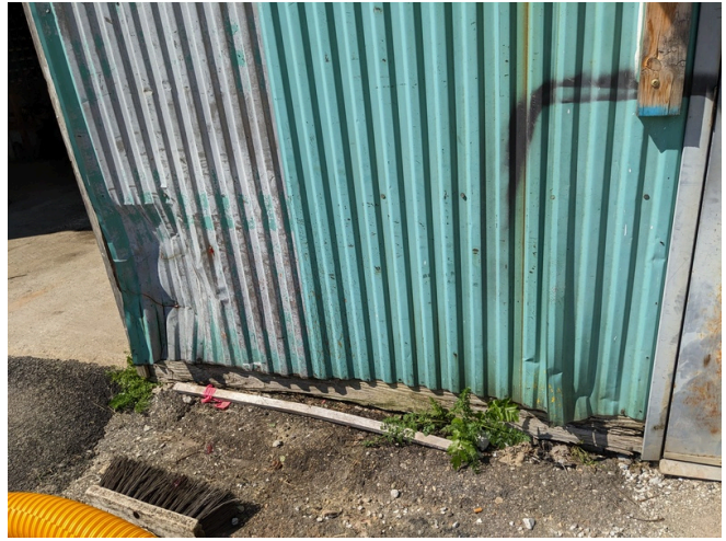
New -South Wall
