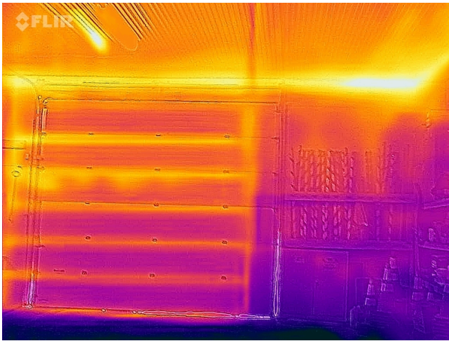
New - IR South Wall Overhead Door in the West Room; Southwest Corner Top Plates
