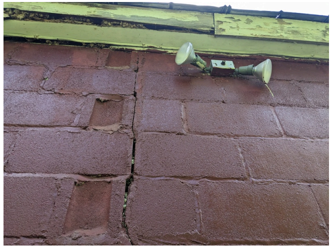
Old - Outside Lighting
