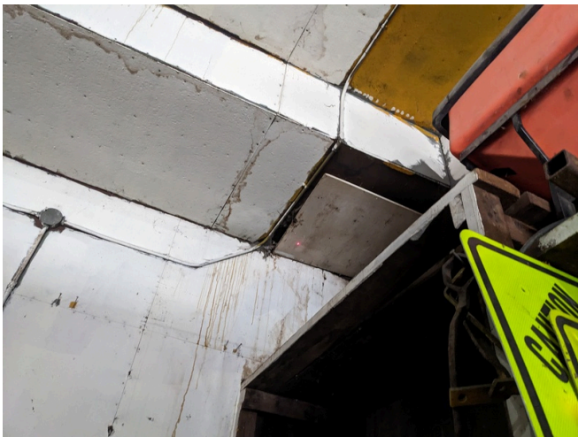
Old - Ceiling is not Sealed
