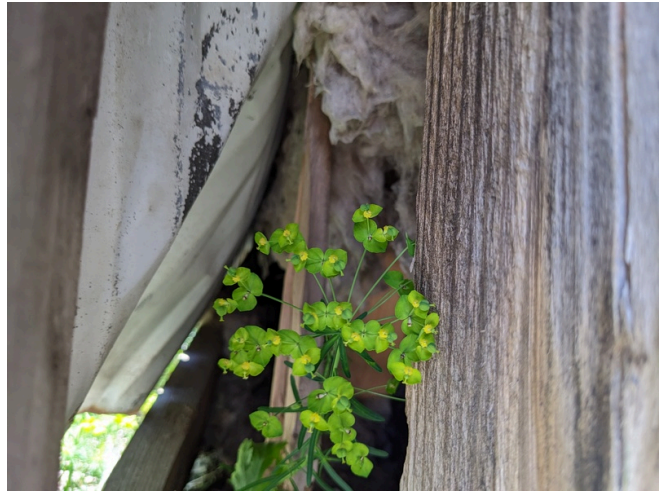
New - Exposed Insulation
