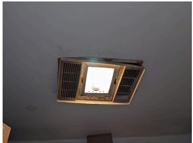
New - Restroom Lighting in the Ceiling Mounted Exhaust Fan
