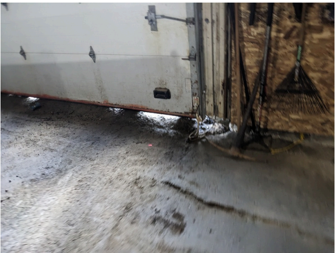
Old - Draft Under the Overhead Doors
